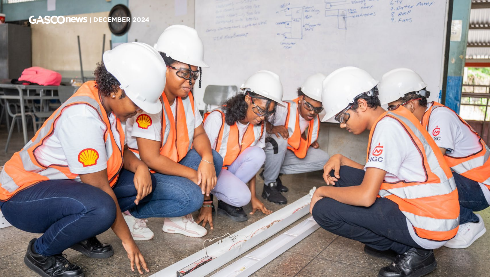
Moruga Secondary students install LED lighting at Basse Terre RC for their green initiative
