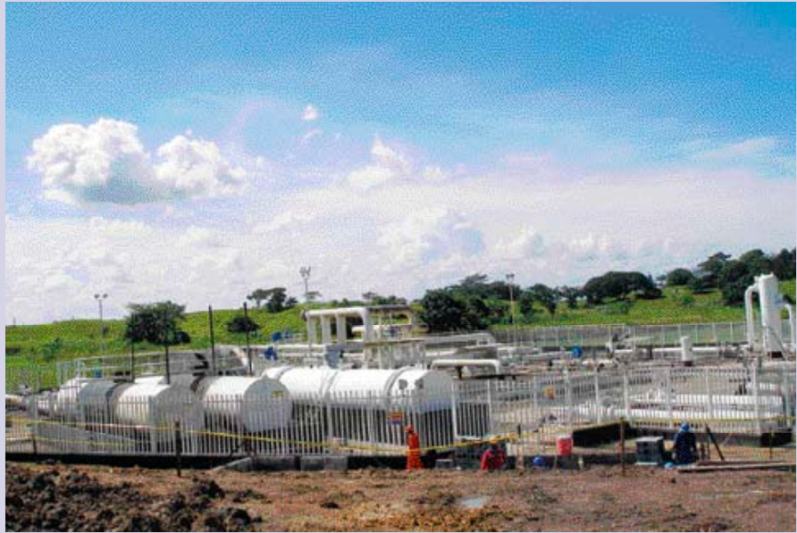
Phoenix Park Valve Station
